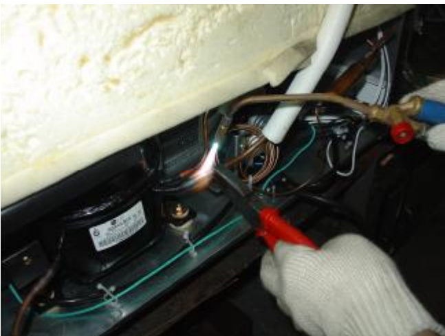
i. 然后，充氮气检此焊点，直到没有气泡产生 Test with towel as charging Nitrogen until there are no bubbles.
