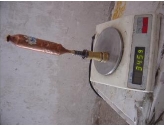
o. 罐装瓶与快装接头相接，压缩机通电 5 分钟以上，注入制冷剂 Connect the canned bottle with the process tube and then compressor work for more than 5 minutes, charge the refrigerant into compressor
