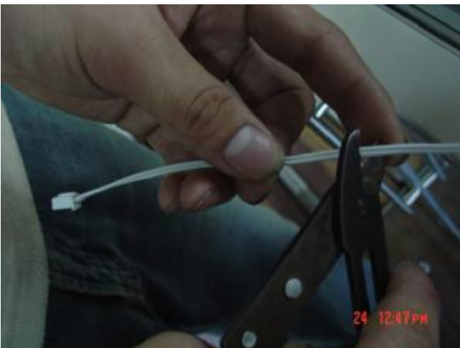
d.重新接上好的接线柱，用胶布隔离捆扎结实 Reconnect a new terminal, and tie it up with rubberized fabric.
